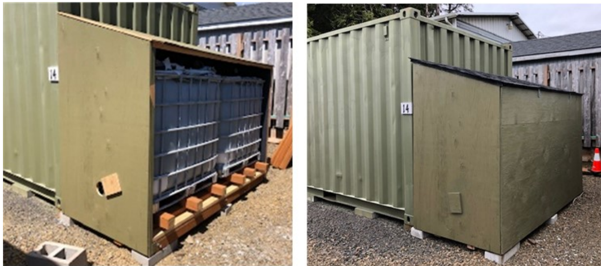
Figure 46: Two 275-gallon Caged Water Containers. Left: shed during construction. Right: finished shed.
